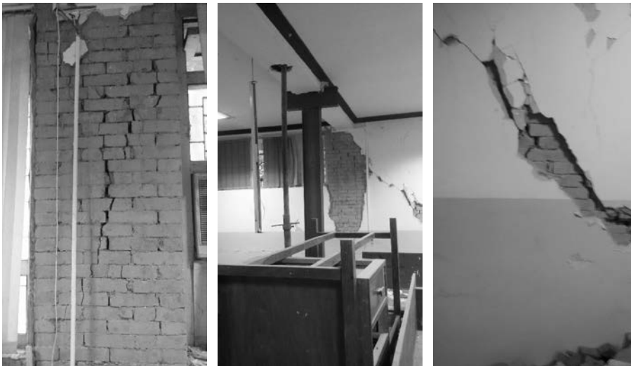
Figure 1: Brick crushing in the masonry piers- outside and inside views
