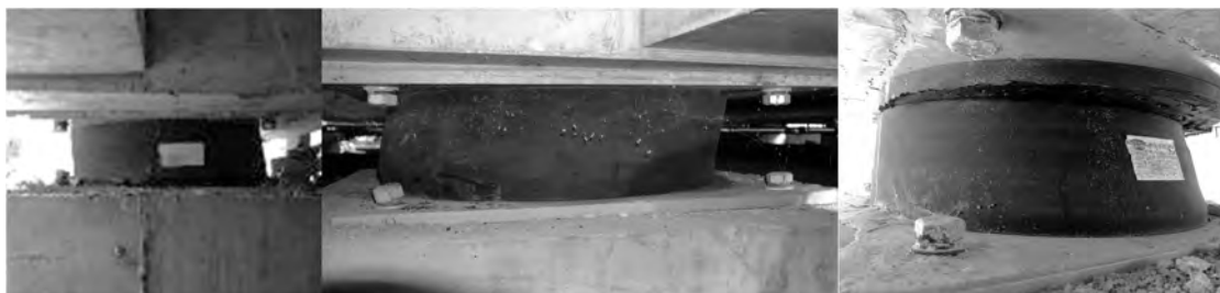
Figure 1 Observed damage to isolators
