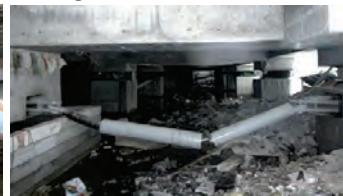
Buckling of damper
