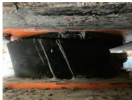
Shear failure of rubber bearing
