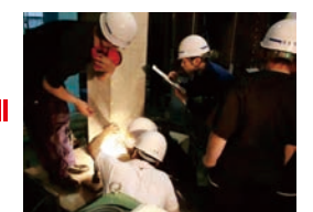
Damage observation in structural tests
